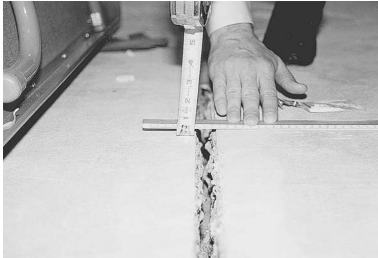
FIGURE 10.2 Damage due to lateral movement.
