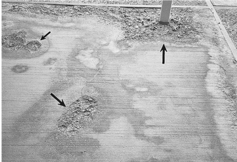
FIGURE 12.3 Concrete patio deterioration, Mojave Desert. The arrows point to deterioration of the concrete surface.
