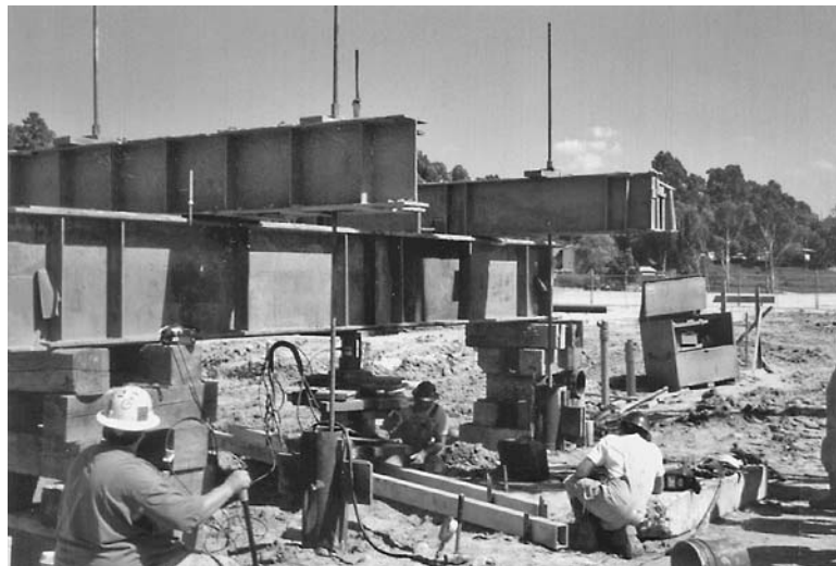
FIGURE 16.34 Pile load tests. The reaction frame has been set up and the hydraulic jack and load cell are in place.
