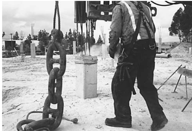
FIGURE 6.10 The prestressed concrete pile at the center of the photograph is the same pile as shown in Fig. 6.9 and has just been driven into place. Note that the cushion blocks of wood have been compressed during the pile driving. The steam emanating from the wood is due to heat generated during the impact with the hammer.
