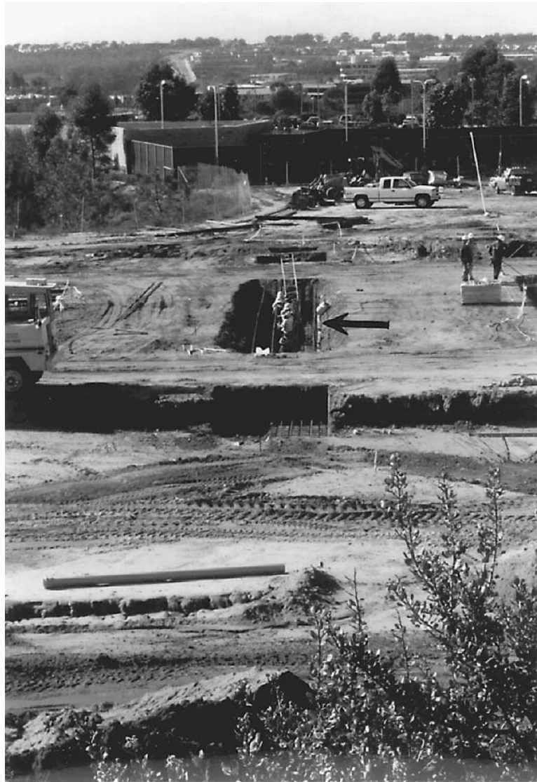
FIGURE 16.3 Installation of steel reinforcement in footings. The arrow points to the workers in the footing excavation in the process of installing the steel reinforcement.
