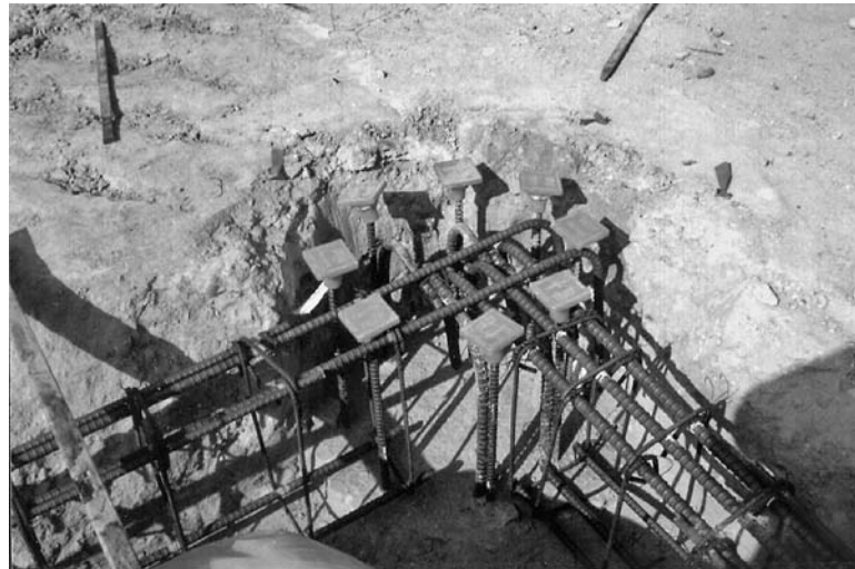
FIGURE 16.16 Corner of the building where the steel reinforcement from the two grade beams has been attached to the steel reinforcement from the pier.
