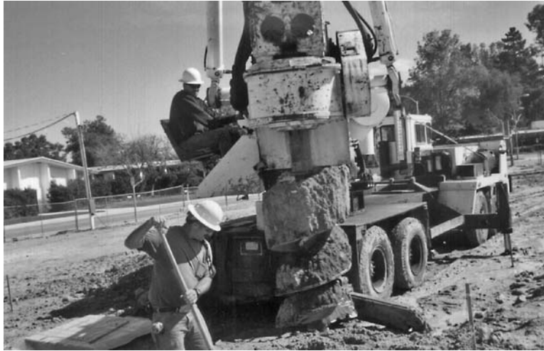
FIGURE 16.11 Close-up of auger being extracted from the ground with soil lodged within its grooves.
