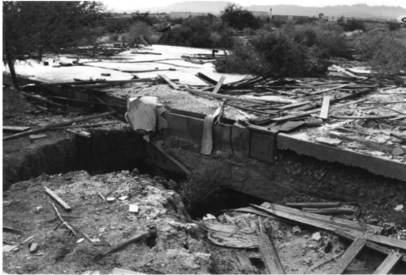
FIGURE 7.18 Ground fissure running underneath a foundation, Las Vegas, Nevada.
