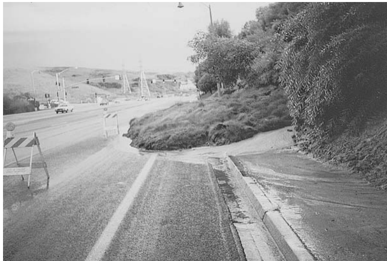
FIGURE 10.14 Partial mobilization of a surficial failure.
