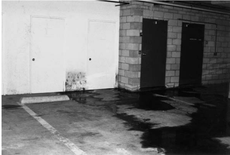
FIGURE 11.21 Photograph of a basement wall subjected to hydrostatic water pressure.
