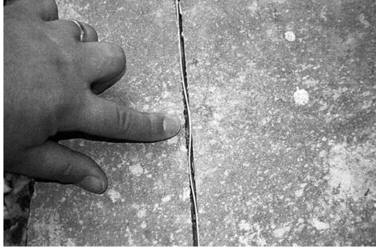
FIGURE 12.14 View of a plastic strip that was used to form a contraction joint. The plastic strip is sometimes referred to as a zip-strip . The gaps that have opened-up on both sides of the plastic strip were caused by drying shrinkage.
