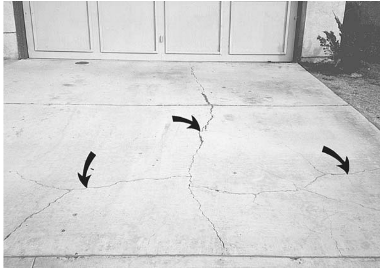
FIGURE 9.31 Driveway cracking due to expansive soil.
