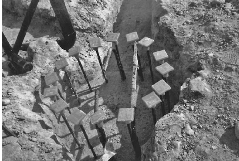
FIGURE 16.13 The pier hole has been filled with concrete. The steel reinforcement from the pier will be attached to the steel reinforcement in the grade beam.
