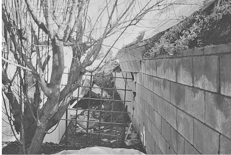
FIGURE 11.7 Collapse of a retaining wall that has a clay backfill.
