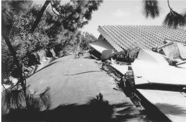
FIGURE 10.31 Laguna Niguel landslide: view of the toe of the landslide where the road has been uplifted 20 ft.
