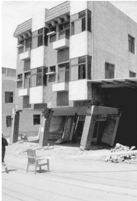
FIGURE 14.1 Damage due to a soft story at the ground floor. The damage occurred during the Chi-chi earthquake in Taiwan on September 21, 1999. (Photograph from the USGS Earthquake Hazards Program, NEIC, Denver.)
