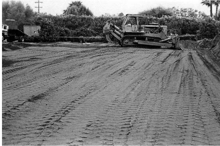
FIGURE 15.3 A lift of fill has been placed and compacted into a dense state.
