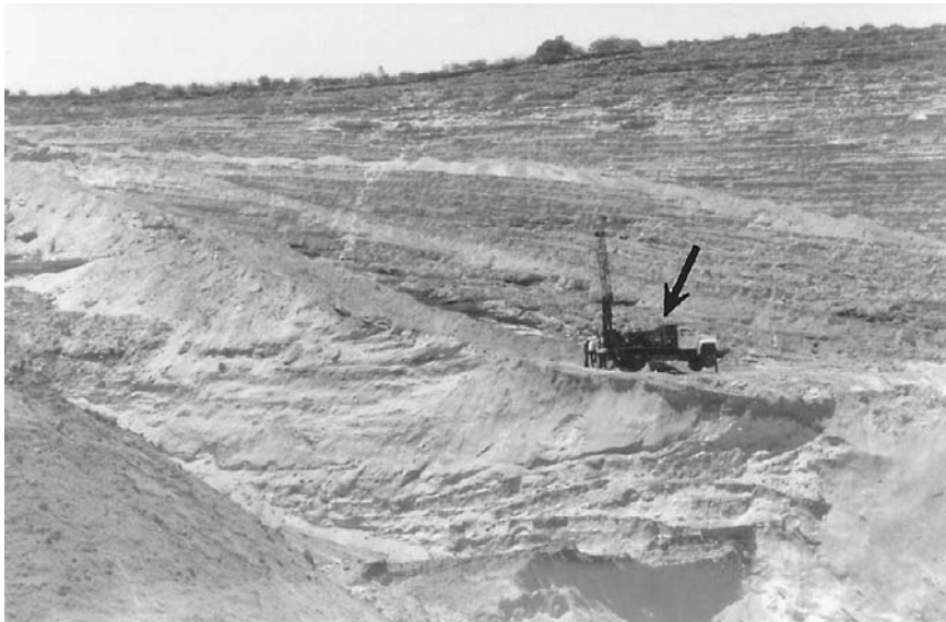
FIGURE 2.28 Access road constructed for subsurface investigation at an open-pit mine (arrow points to bucket auger drill rig).
