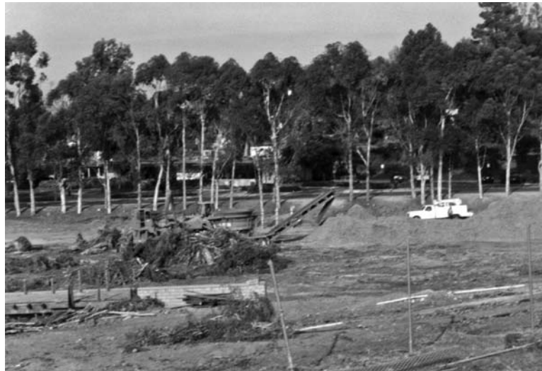
FIGURE 15.2 A large mechanical grinder has been brought to the site and the trees and brush are being ground-up into wood chips. The wood-chips will be removed from the site and then recycled.
