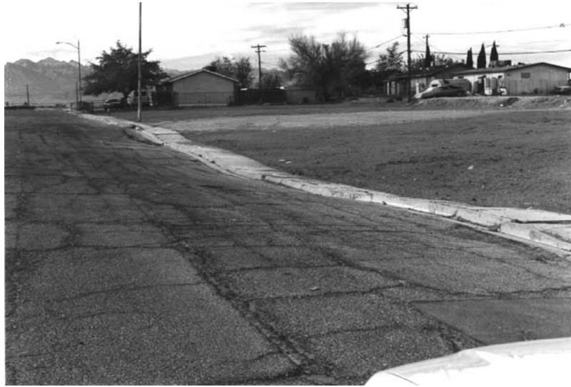
FIGURE 7.20 Settlement of the street and sidewalk due to ground fissures, Las Vegas, Nevada.
