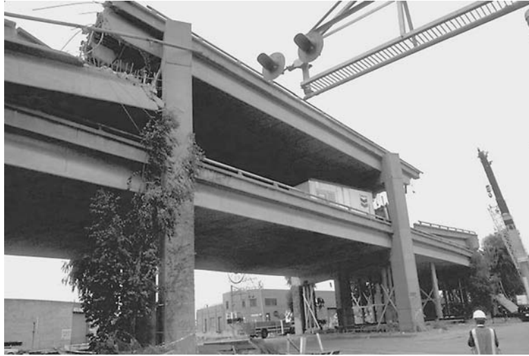
FIGURE 13.14 Another close-up view of the collapse of the Cypress Street Viaduct caused by the Loma Prieta earthquake in California on October 17, 1989. (From USGS.)
