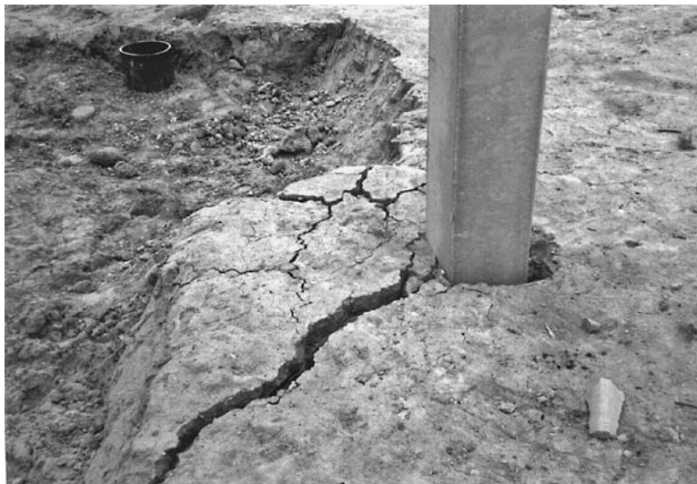
FIGURE 16.24 Lateral displacement of a prestressed concrete pile during the driving operations.
