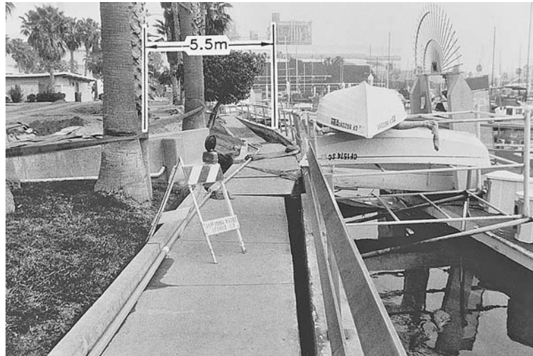
FIGURE 13.19 Damage to a marine facility caused by the California Northridge earthquake on January 17, 1994. (From Kerwin and Stone, 1997; reprinted with permission from the American Society of Civil Engineers.)
