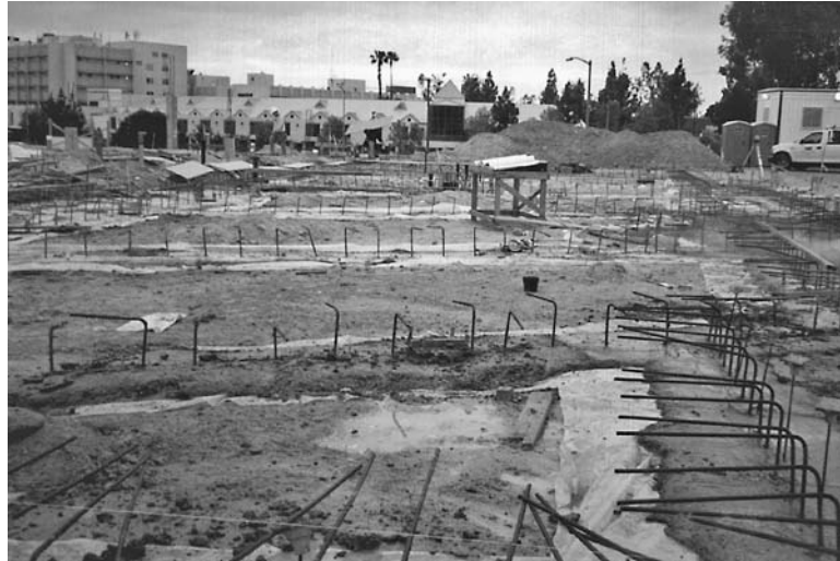
FIGURE 16.17 The concrete for the grade beams has been placed. The steel reinforcement from the grade beams will be attached to the steel reinforcement in the floor slab.
