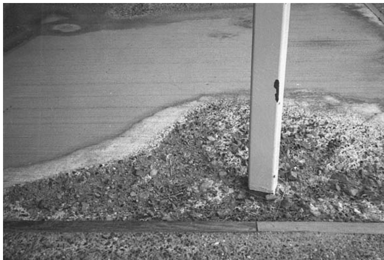
FIGURE 12.4 Concrete patio deterioration, Mojave Desert (note the salt deposits and deterioration of the concrete surface).
