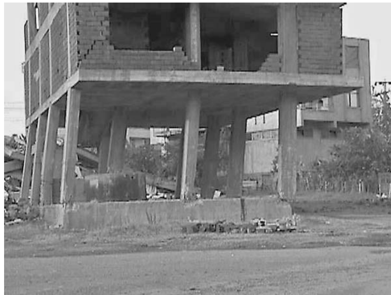
FIGURE 14.4 Damage caused by a soft story at the first-floor level. The damage occurred during the Kocaeli earthquake in Turkey on August 17, 1999. (Photograph by Mehmet Celebi, USGS.)
