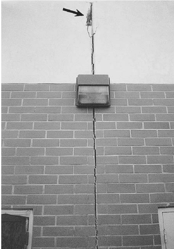
FIGURE 10.3 Joint separation between wall panels.
