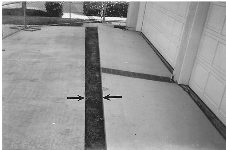
FIGURE 10.38 Laguna Niguel landslide: head of the landslide showing lateral movement of the entire house. (Note: The distance between the arrows indicates the amount of lateral movement.)
