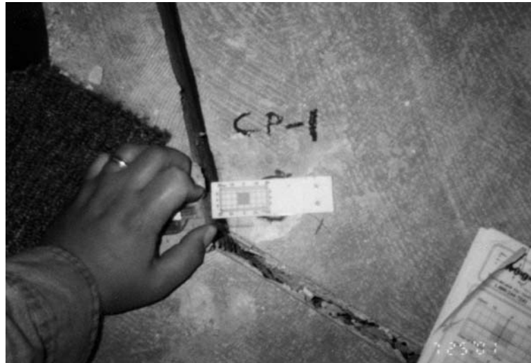
FIGURE 12.15 About 1 in. (25 mm) opening of a contraction joint due to slope movement that pulled apart the foundation at the contraction joints. A crack monitoring device has been placed across the contraction joint.
