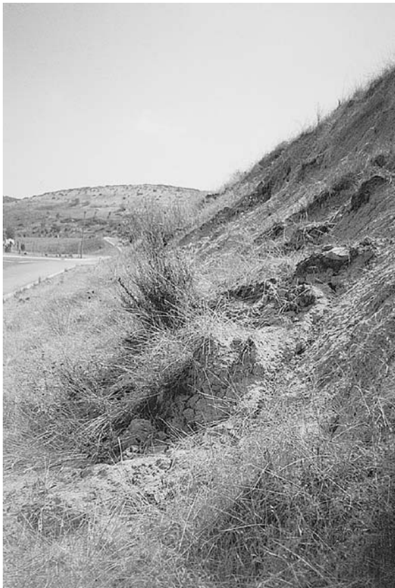
FIGURE 10.12 Surficial failure, cut slope for road.
