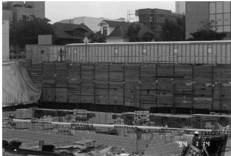
FIGURE 11.19 Temporary steel I-beam and wood lagging retaining wall having tieback anchors. The temporary retaining wall is being used to support the excavation during the construction of the foundation.
