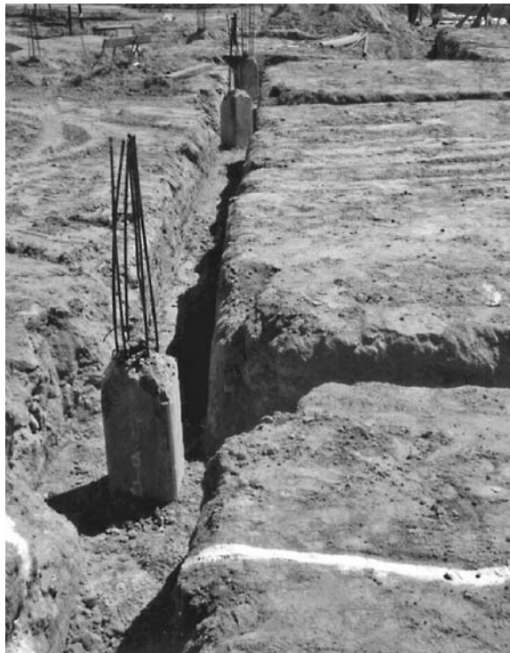
FIGURE 16.26 Prestressed concrete piles have been installed and the excavations for the pile caps and grade beams are complete. The strands at the top of the pile will be connected to the steel reinforcement in the pile cap and grade beam.
