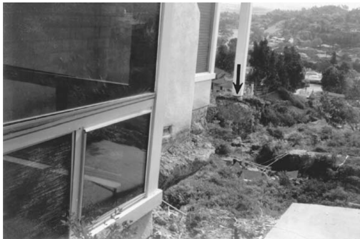
FIGURE 10.36 Laguna Niguel landslide: head of the landslide showing another house with a portion suspended in mid-air. (Note: The arrow points to a column and footing that are suspended in midair.)
