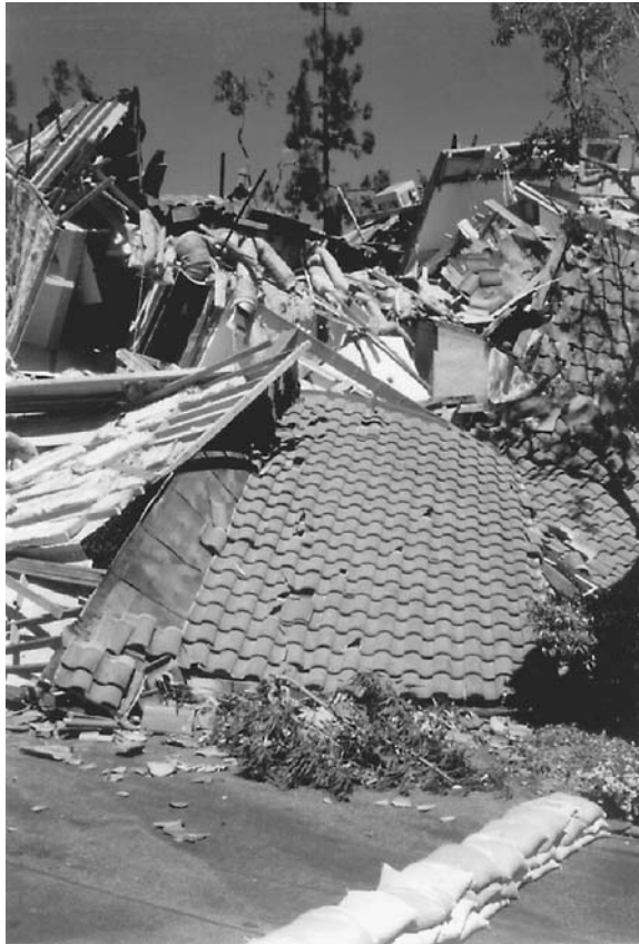
FIGURE 10.33 Laguna Niguel landslide: view of damage at the toe of the landslide. The landslide has crushed the buildings located in this area.
