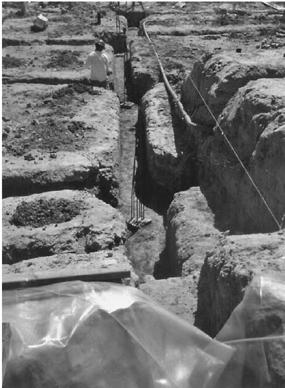
FIGURE 16.28 The excavation for the grade beams is complete and the top of the prestressed piles are trimmed so that they are relatively flush.
