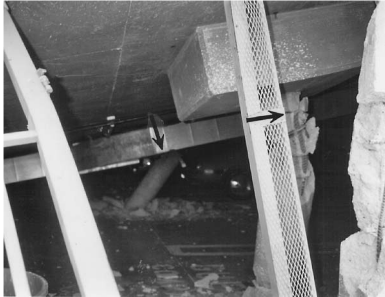
FIGURE 14.3 View inside the collapsed first floor parking garage (the arrows point to the columns). The building collapse occurred during the Northridge earthquake in California on January 17, 1994.
