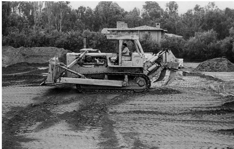
FIGURE 15.9 The bulldozer is in the process of spreading out a layer of fill for compaction.
