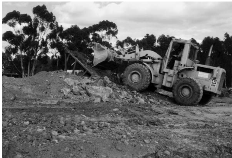
FIGURE 15.6 A loader is in the process of depositing material on top of the screen in order to separate the large size rock fragments.
