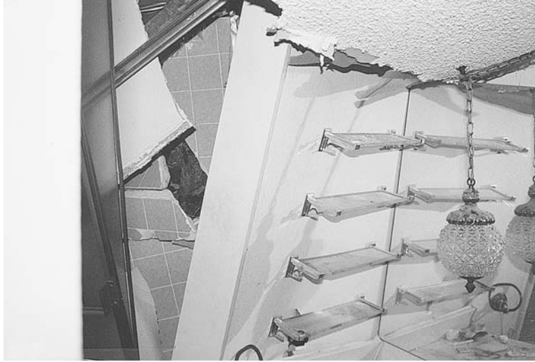
FIGURE 10.7 Damage to bathroom.
