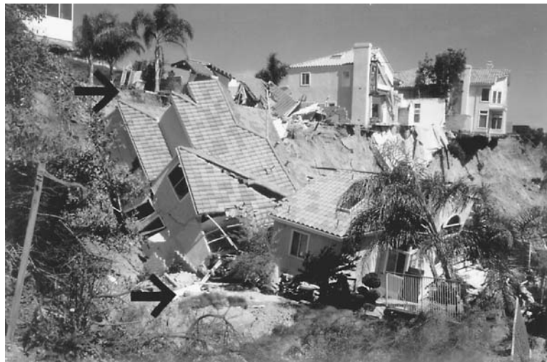
FIGURE 10.34 Laguna Niguel landslide: head of the landslide. ( Note: The vertical distance between the two arrows is the distance that the landslide dropped downward.)
