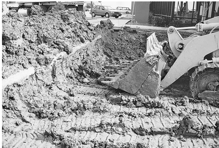
FIGURE 15.16 Pumping of clay subgrade during construction.
