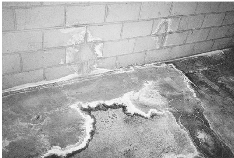
FIGURE 11.23 Two views of groundwater migration through basement walls at a condominium complex in Los Angeles, California.
