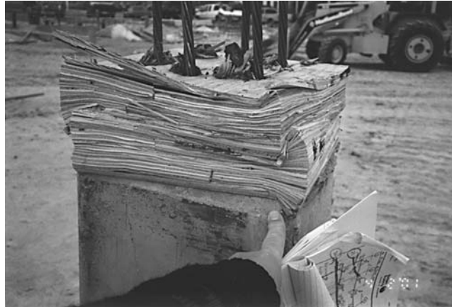
FIGURE 6.11 Close-up view of Fig. 6.10. The wood cushion blocks have been crushed together during the pile driving operation.
