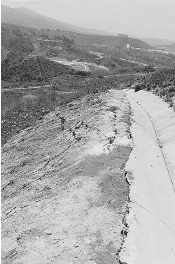
FIGURE 10.15 Ground cracks associated with incipient surficial instability.
