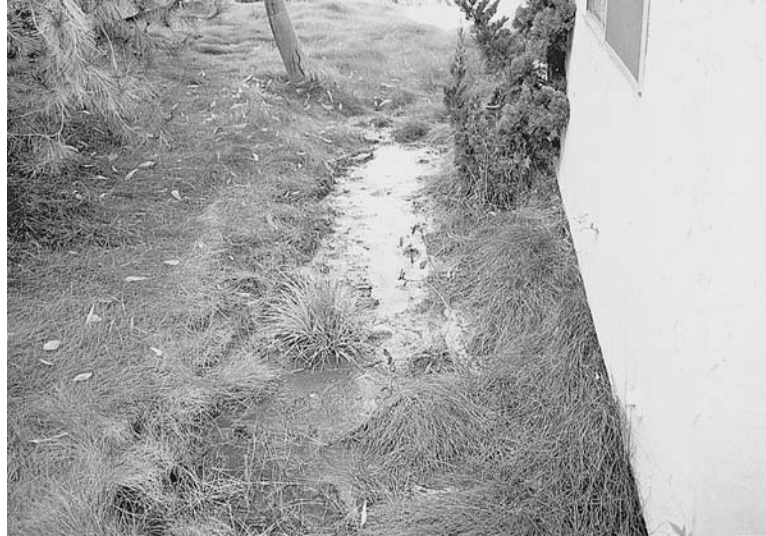
FIGURE 12.21 Poor surface drainage at a condominium complex.
