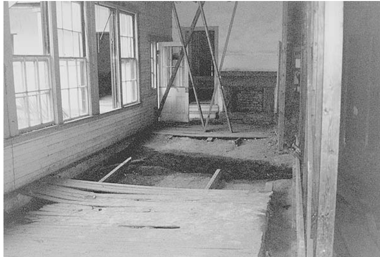
FIGURE 12.9 Drainage beneath parlor.
