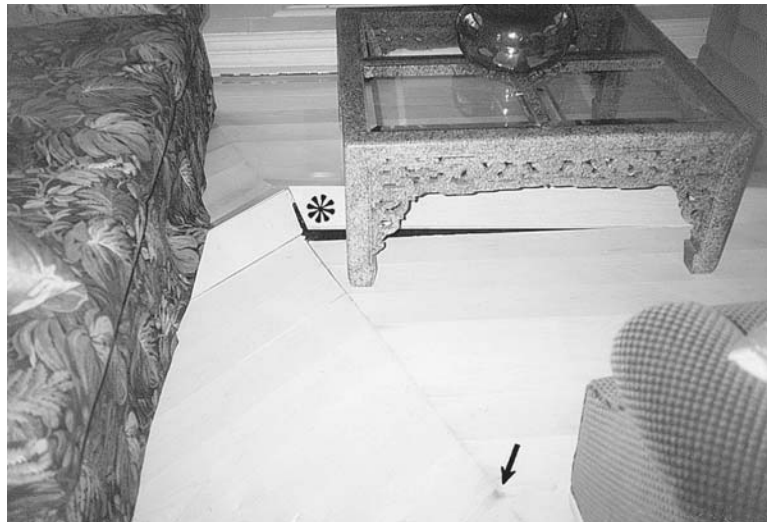
FIGURE 12.17 Damage to wood flooring. The arrow points to a moisture stain and the asterisk indicates upward warping of the wood floor.
