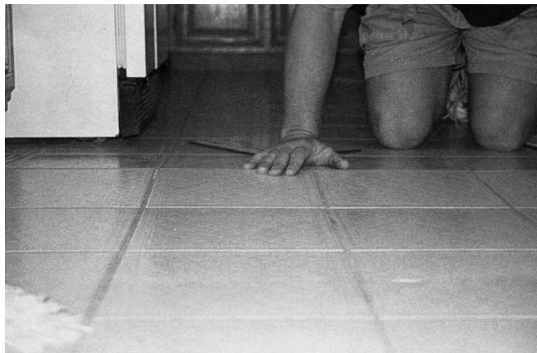
FIGURE 12.18 Uplift of floor tile due to moisture migration through a crack in the slab-on-grade foundation. The floor tile absorbed moisture and expanded, resulting in the uplift shown in the photograph.
