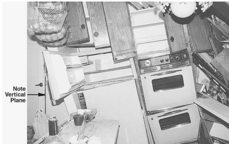
FIGURE 10.6 Damage to kitchen area.
