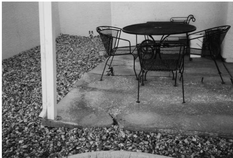
FIGURE 12.1 Sulfate attack of a concrete patio.
