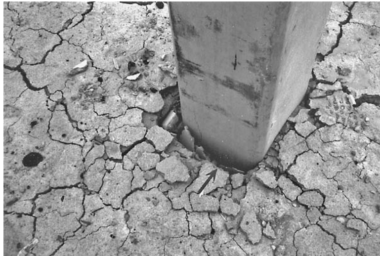
FIGURE 16.25 This prestressed concrete pile struck an underground obstruction, displaced laterally, and broke near ground surface. The arrow points to the location of the breakage.
