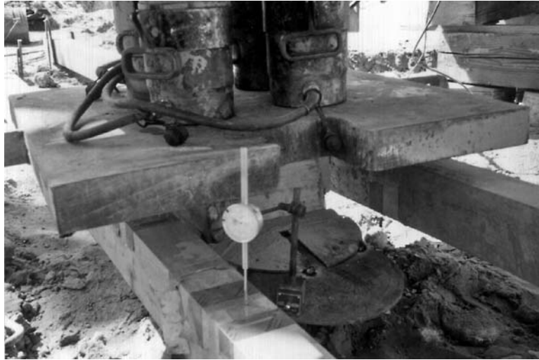
FIGURE 16.35 Pile load tests. This photograph shows one of the dial gauges that are used to record the vertical displacement of the top of the pile during testing.
