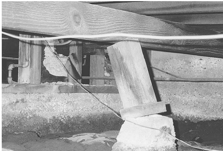
FIGURE 9.23 Expansive soil damage of a raised wood floor foundation. Note the wet condition of the soil in the crawl space.
