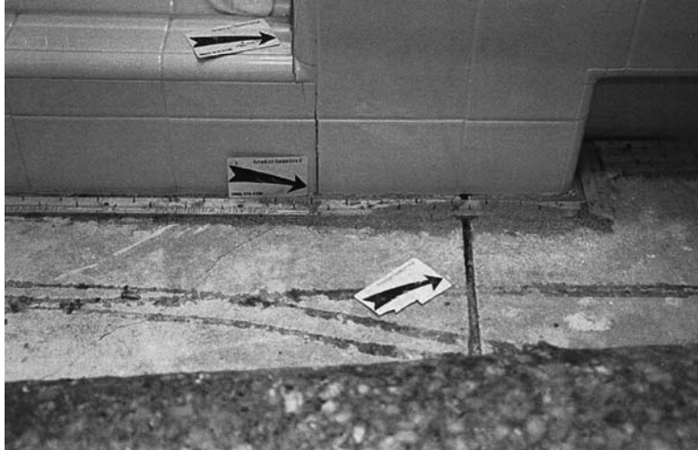
FIGURE 12.16 The opening of a contraction joint (lower arrow) has resulted in the cracking of shower tiles (upper arrow) that span the contraction joint.
