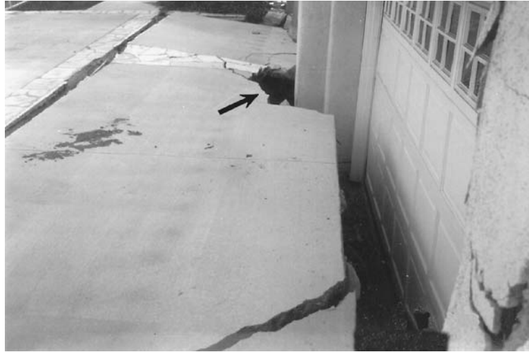
FIGURE 10.37 Laguna Niguel landslide: head of the landslide where a house has dropped downward. (Note: The arrow points to the area where the house foundation has punched through the driveway on its way down.)
