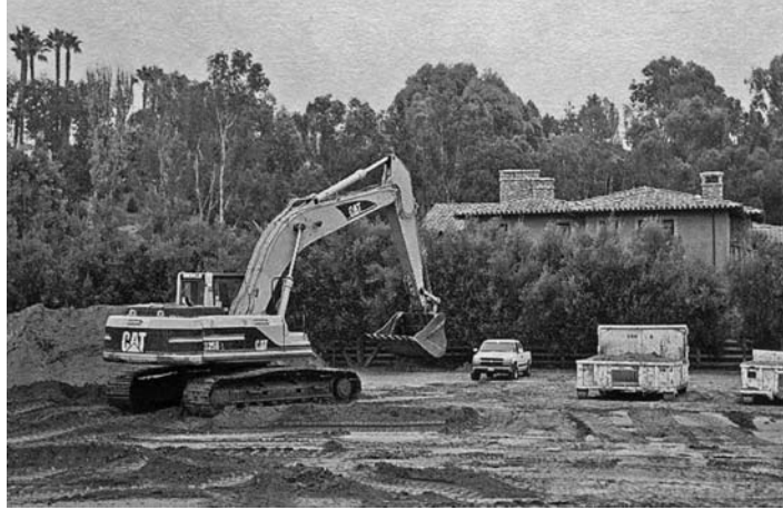
FIGURE 15.12 The excavator is ideally suited to excavating narrow trenches for the construction of utilities such as storm drain lines and sewer lines.
