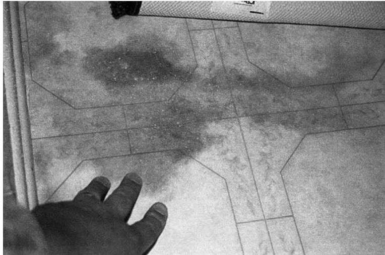
FIGURE 12.19 Linoleum discoloration due to moisture migration through a crack in the slab-on-grade foundation. The moisture accumulated beneath the linoleum at the location of the slab crack and caused the darkening of the linoleum as shown in the photograph.
