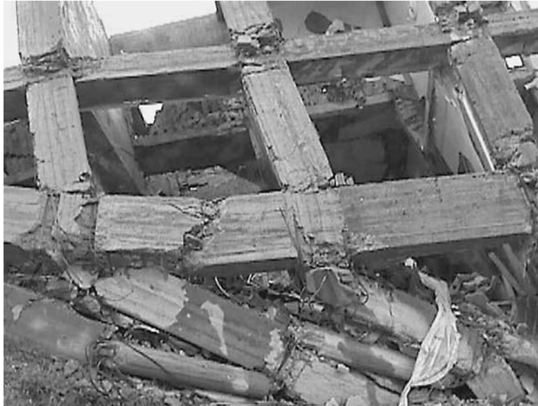
FIGURE 14.5 Building collapse caused by a soft story at the first-floor level. The damage occurred during the Kocaeli earthquake in Turkey on August 17, 1999. (Photograph by Mehmet Celebi, USGS.)
