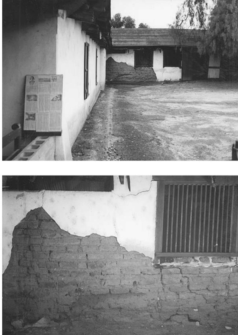
FIGURE 12.8 Deterioration of adobe. The lower photograph is a close-up view of the upper photograph. Note that the individual adobe blocks are visible in the lower photograph.
