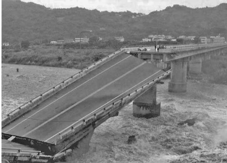
FIGURE 13.5 Collapsed bridge north of Fengyuen caused by surface fault rupture associated with the Chi-chi (Taiwan) earthquake on September 21, 1999. (Photograph from the USGS Earthquake Hazards Program, NEIC, Denver.)
