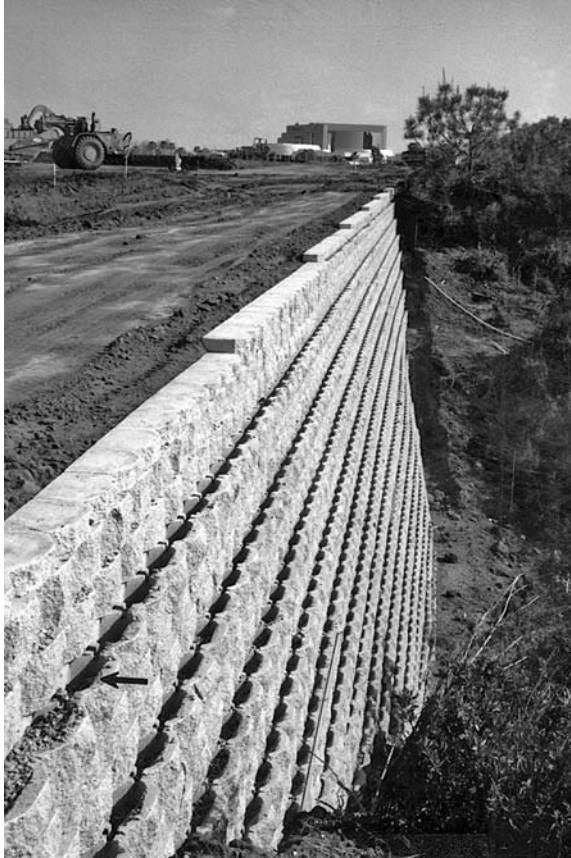
FIGURE 11.11 Final constructed condition of the mechanically stabilized earth retaining wall. The arrow points to an opening in the wall facing element that can be used to establish vegetation on the wall face.
