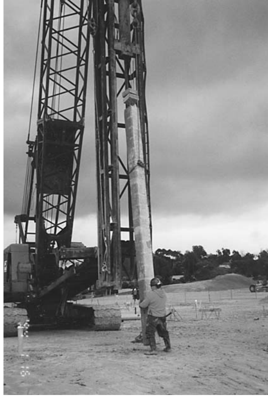
FIGURE 6.9 A prestressed concrete pile is being hoisted into place for driving. Wood blocks have been placed at the top of the pile to cushion the impact of the drive hammer and prevent damage to the top of the pile.
