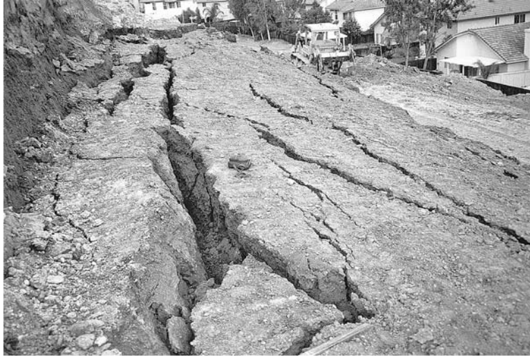
FIGURE 16.1 Slope failure during the grading of a site. The backpack located in the middle of the photograph provides a scale for the size of the ground cracks.
